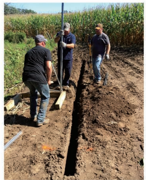
Site installation at Daugs Road. From left: Matt Komiskey, Brian Goepfert, and Dustin Ladd.
