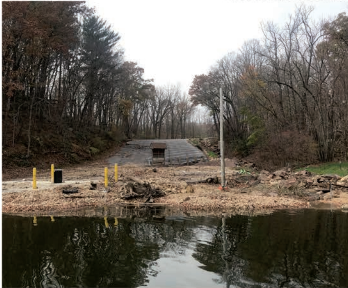
Flood damage to section 11 boat landing.
